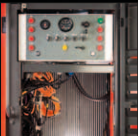
Practical location for electrical cabinet
