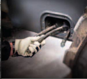
Centralised oil removal – hoses to facilitate oil changing
